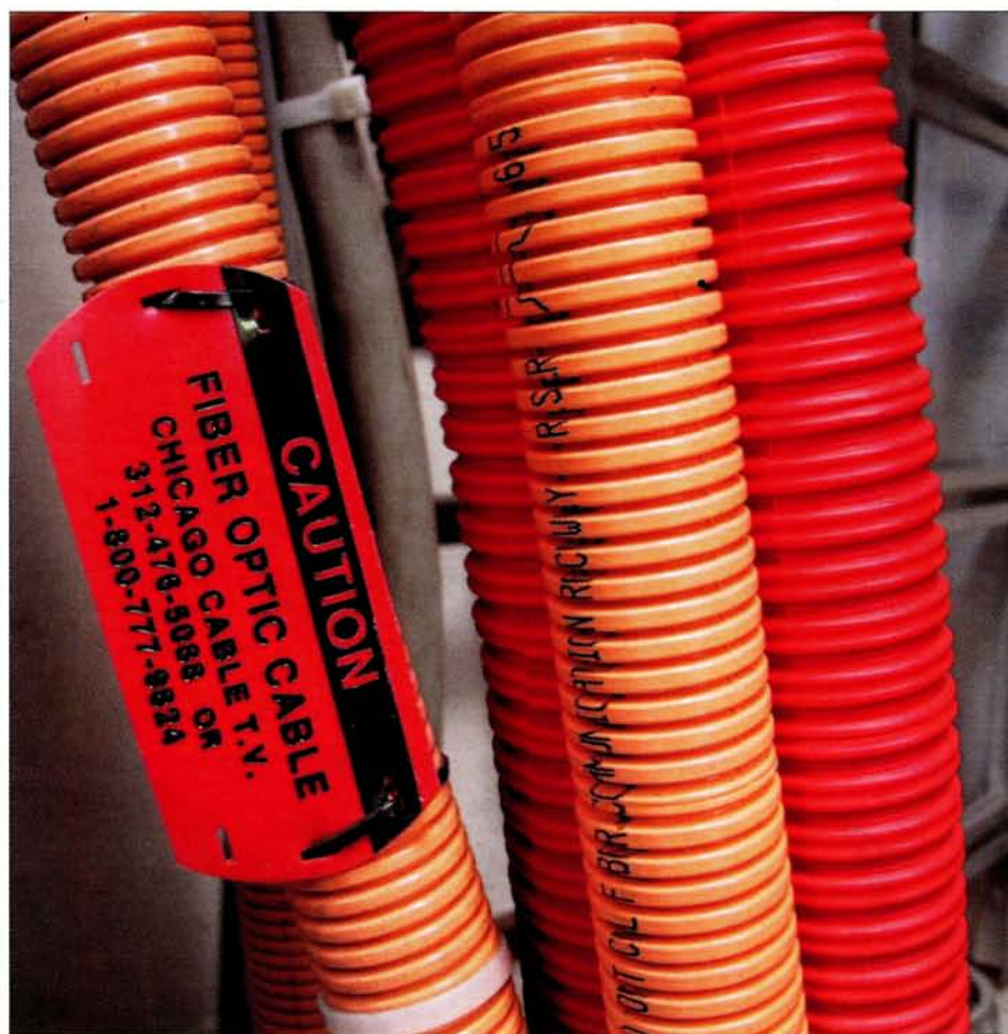
Optical cables at Chicago's StarLight™ Internet exchange. StarLight is the emerging optical component of the National Science Foundation-funded STAR TAP™ international interconnection point for advanced research and education networks. (Electronic Visualization Laboratory, University of Illinois, Chicago.)
